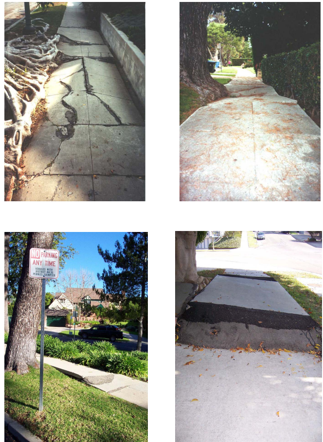
Fig. 1. Broken sidewalks in Los Angeles
