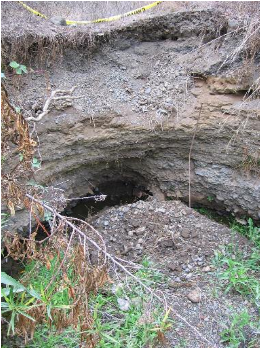
FIGURE 17. View of bank downstream of Area IV. Bank erosion is evident next to north channel just before joining south channel. Photo taken by Colin Dudley on November 3, 2005.
