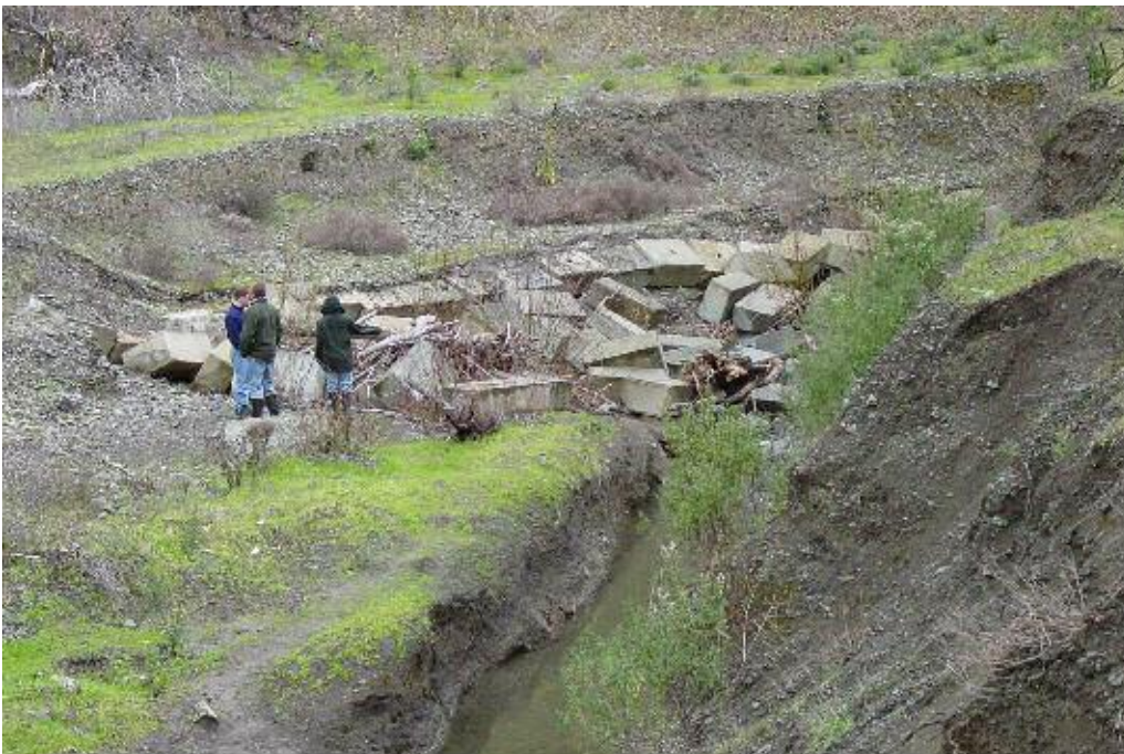
FIGURE 4. View upstream of Area IV prior to restoration in 2002. Concrete blocks were placed along the right bank to prevent bank erosion. Unknown photographer, image courtesy of SCWA.
