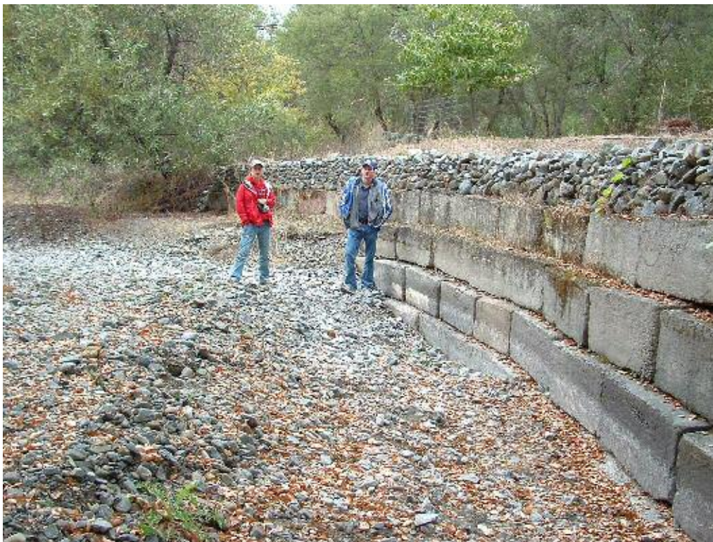
FIGURE 6. Concrete block wall on left bank of channel, downstream of Crocker Creek Dam removal site. Rocks on top of wall appear to be in place to raise effective height. Looking upstream. Photo taken by Alicia Gilbreath on November 3, 2005.
