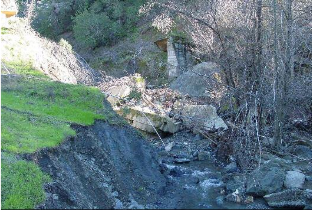
FIGURE 1. View upstream of failed Crocker Creek Dam in 2002. Unknown photographer, image courtesy of SCWA.
