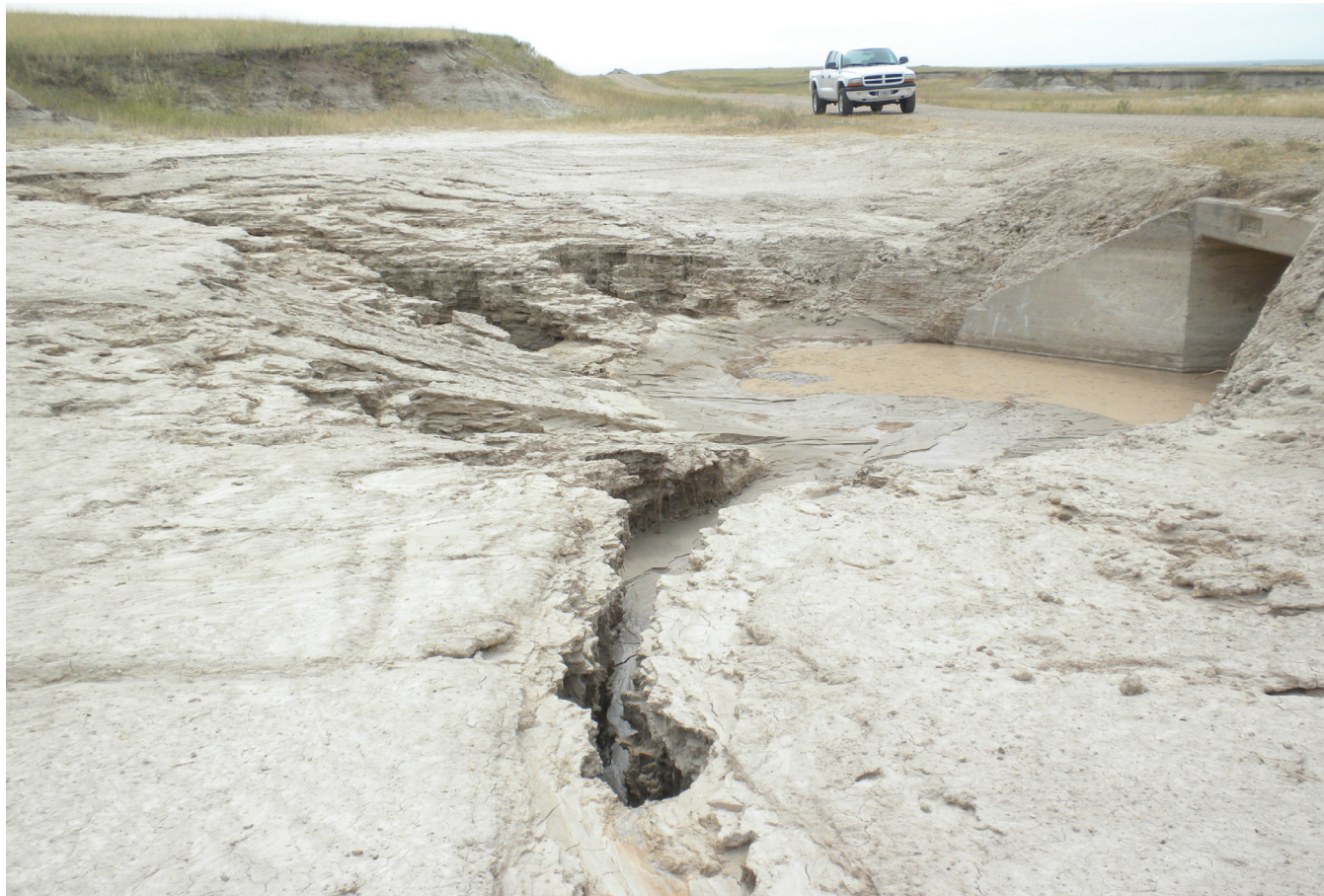
FIGURE 1. ABOVE A box culvert and associated drainage along Old Interior Road that was cleaned and shaped by the Maintenance Division in 2011. A system of box channels was created by subsequent precipitation. BELOW The same drainage system in 2023. The box channels are still present but erosion at the inlet of the culvert has abated, allowing vegetation to proliferate.
