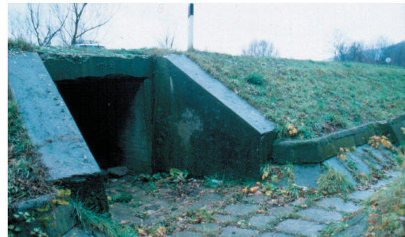
Photo 10. Square culvert opening with concrete fence set up for directing amphibians into the culvert.
