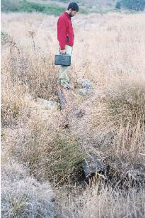
Figure 5. David Shaw standing on remnants of old bridge and culverts on the North Tributary #2.
