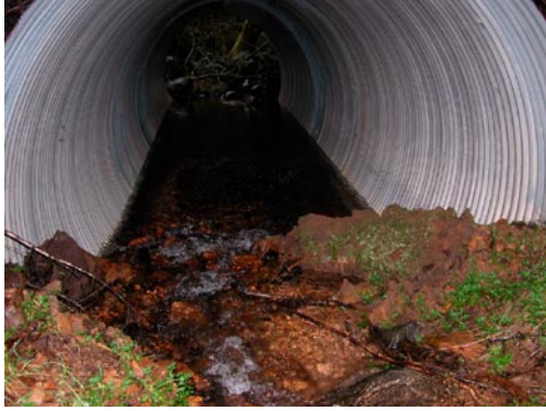
Fig. 14. Design/Construction Problem – eliminated streambed material.
