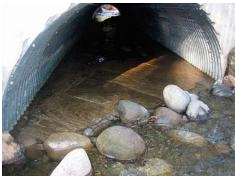
Fig. 16. Construction Problem – Supply of incorrect streambed: contract or administration?
