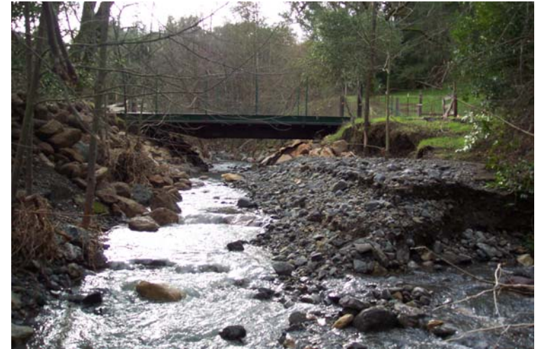
January 2006 – showing sediment deposition and rock repair on bank
