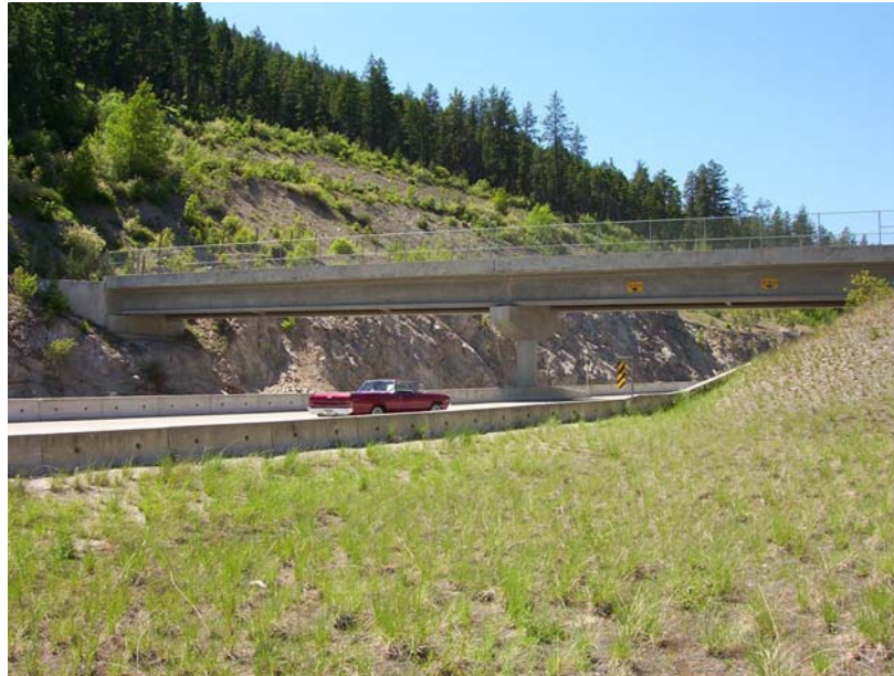
Figure 20. Trepanier wildlife overpass on Okanagan Connector
