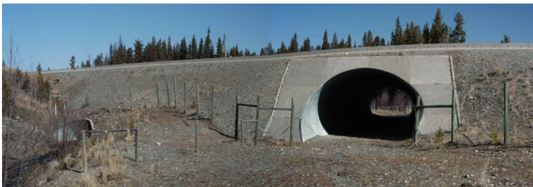
Figure 8. Wildlife underpass designed for deer on the Okanagan Connector (early 1990’s)
