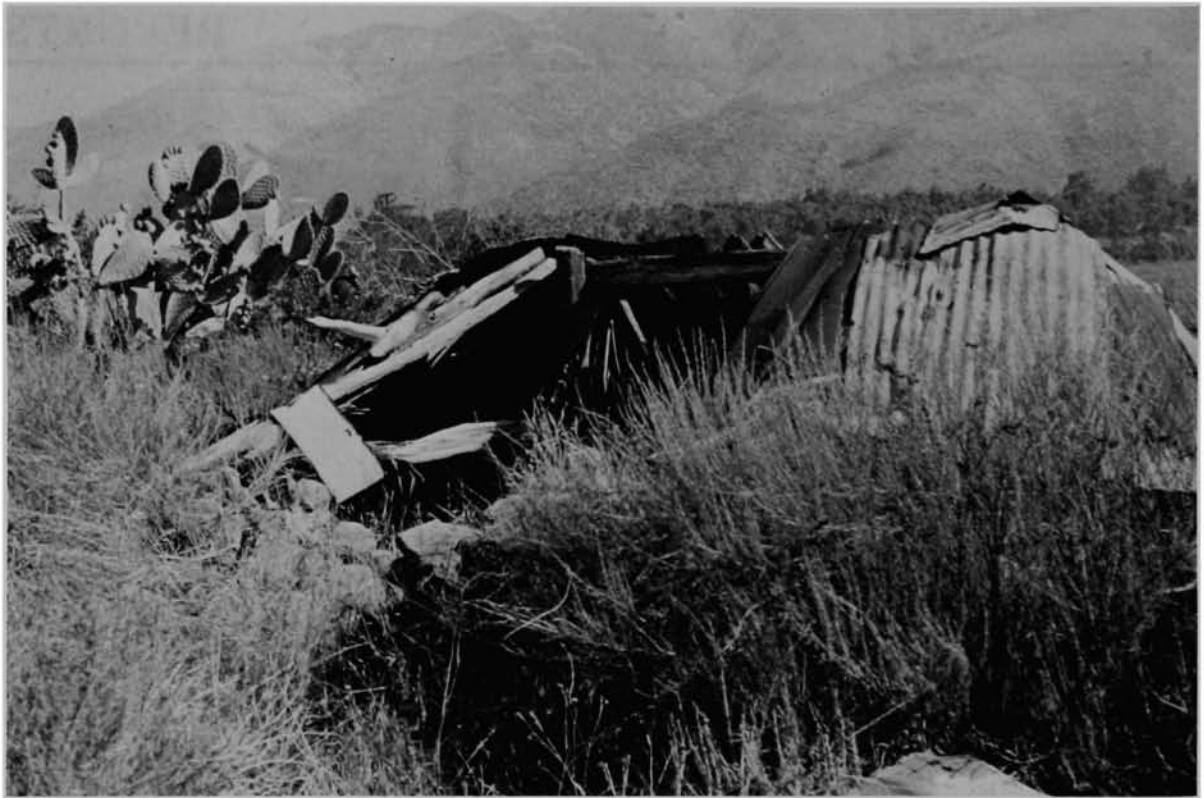
Fig. 2. Photograph showing construction detail and condition of the Pauma sweat house in 1958.
