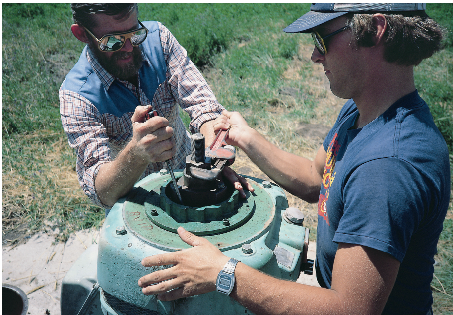
Adjustments to impellers, made by turning the nut at the top of the pump shaft, can improve pump efficiency. But that may not necessarily translate into energy savings, unless operating time is reduced.
