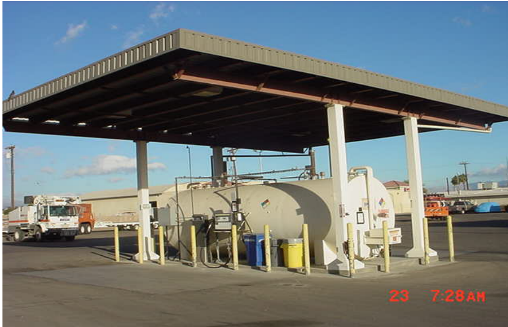
Figure 6-2. Fuel Tank Used at the Indio Maintenance Yard
