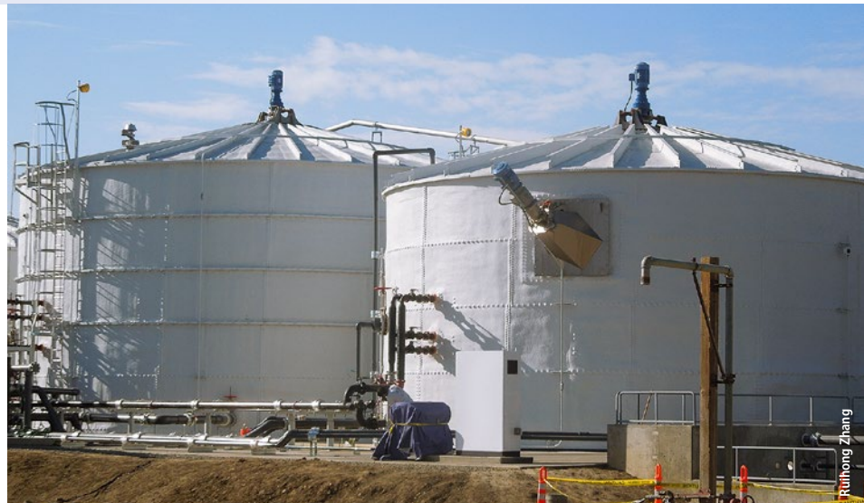
On the UC Davis campus, anaerobic digesters break down food waste and manure and generate biogas.
