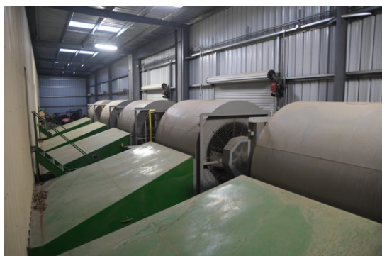
Rear fan room of the in-bin walnut drying facility, where the centrifugal fans and burner assemblies provide heated air to the drying bins. The angled green bin tops (burners) connect to individual ducts leading to each blower. Roll-up doors along the back wall control outdoor air intake and serve as the main mechanism for air recirculation (AR) during drying. Photo: Alice Dien.
